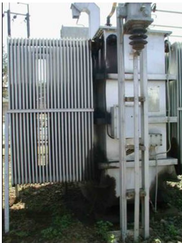
P4: 132 KVA Power transformers at Kivungi Substation, Moshi
