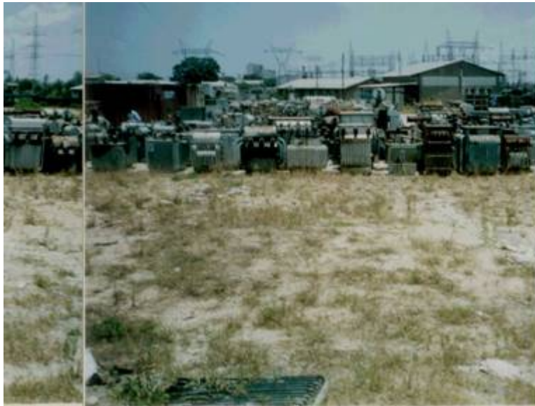
P2: Out of service transformer stored outside the Ubungo Central Workshop
