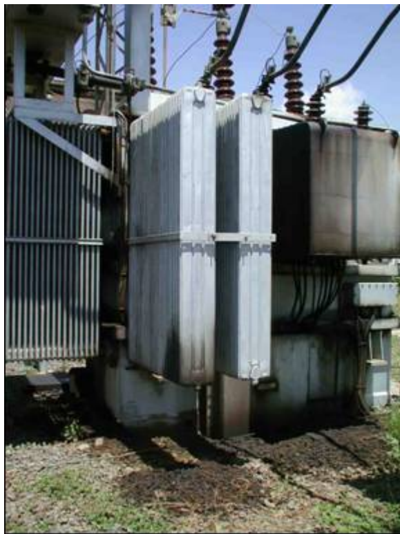
P3: Power transformer at a substation located at the Old power station Arusha, Unga Limited area
