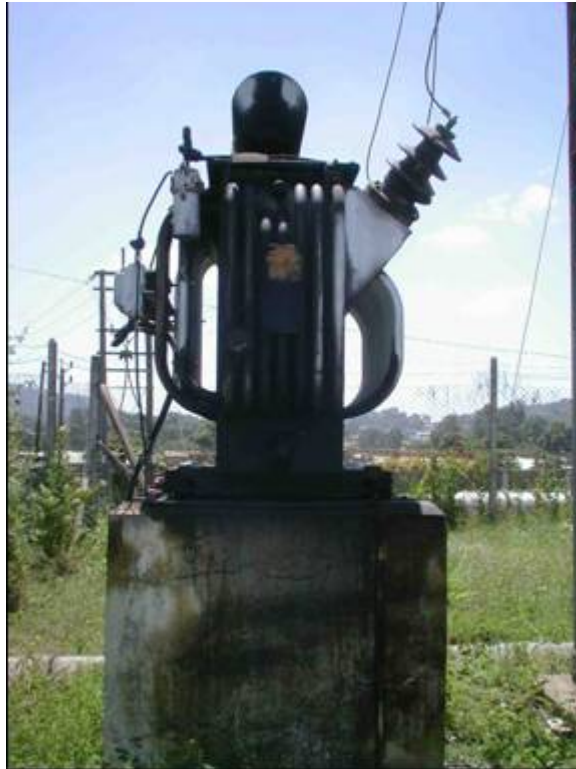
P1: A distribution transformer at a substation near TBL in Arusha
