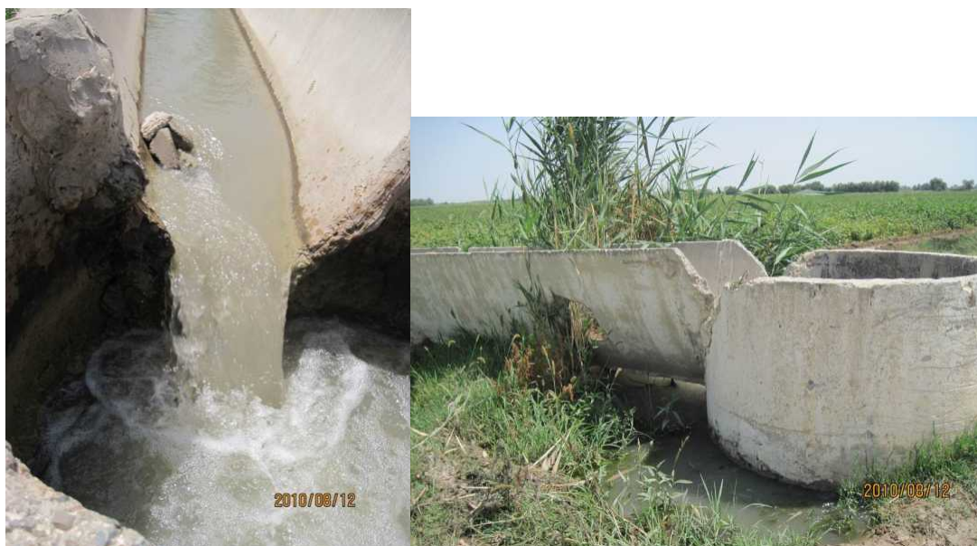
Photo by D. Zainutdinova. Deteriorated drainage collectors in Sarbadinskiy district of Syrdaryinskaya oblast
