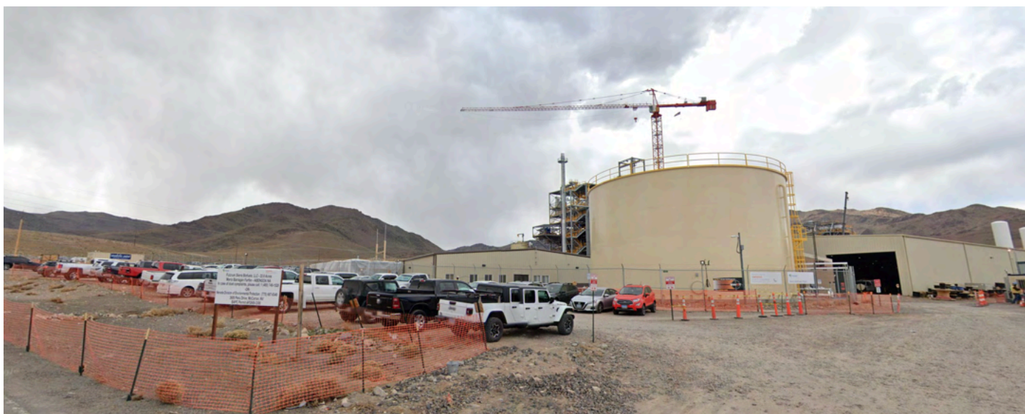
Fulcrum Sierra Biofuels plant in McCarran, Nevada. Source: Google Street View
