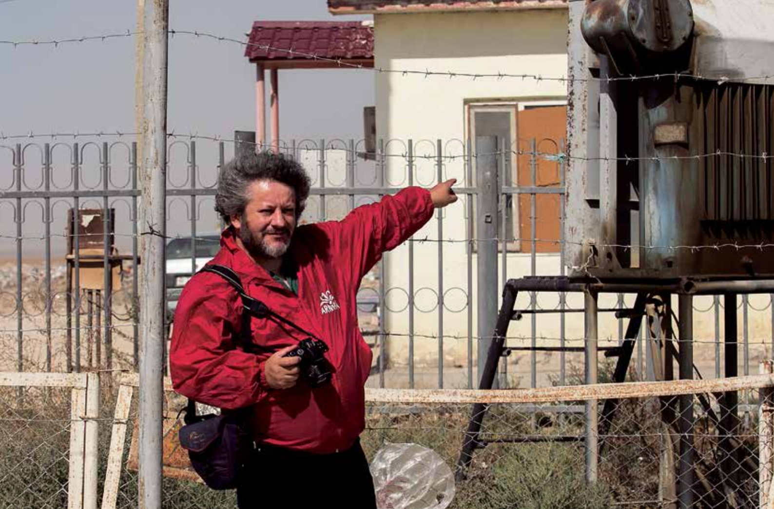
An obsolete leaking transformer at the entrance of the landfill in Baskuduk, north from the sampling site.
