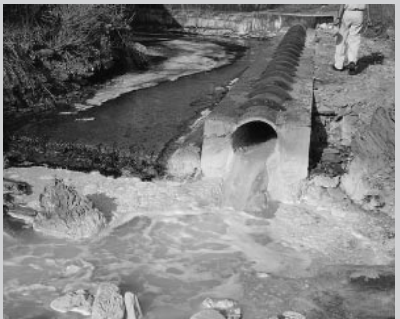
KCIL's effluent discharge pipeline into Donki Nala
