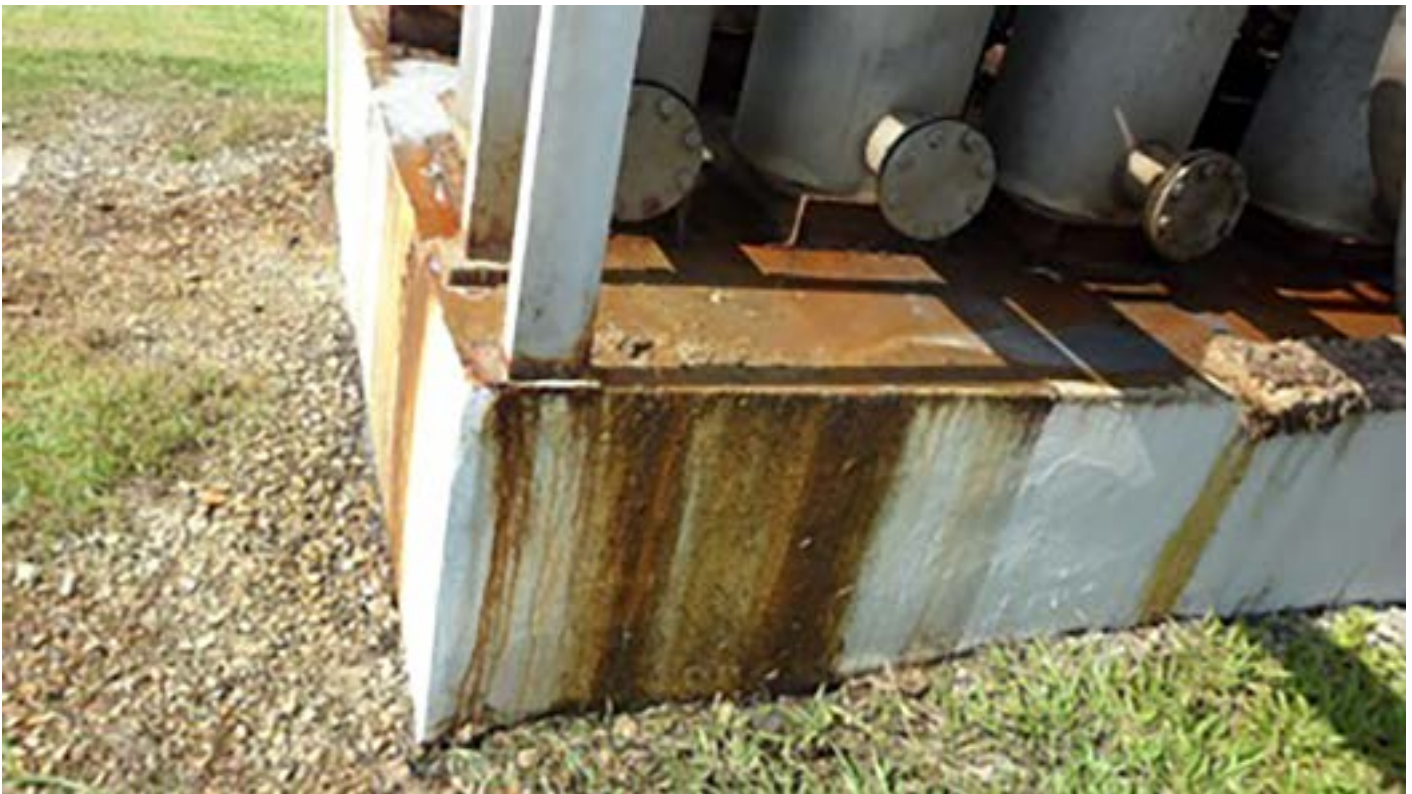
A leak from a water screen circulation pump of a painting process, causing wastewater to leak out.
