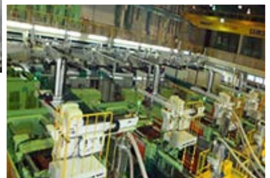
No local exhaust system installed in the injection molding process at Samsung's mobile phone factory in Bac Ninh, Vietnam, resulting in the release of toxic chemicals.
