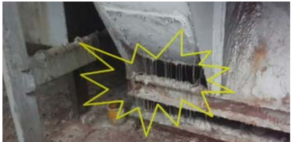
Activated carbon tower at a Samsung Electronics supplier shows failure to periodically replace activated carbon.
