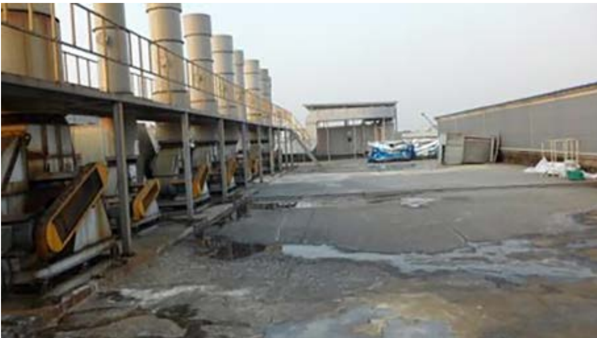
Painting process wastewater flowing out of the air pollution control facilities at the Bac Ninh plant.
