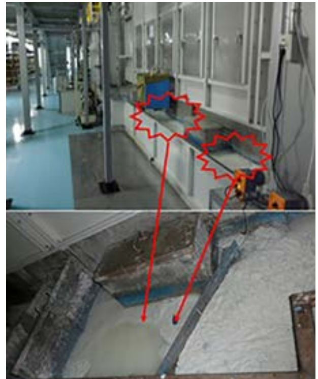
Failure to install a local exhaust system in the paint spray wastewater treatment area of the painting process at Samsung's Bac Ninh factory in Vietnam results in the release of toxic chemicals.
